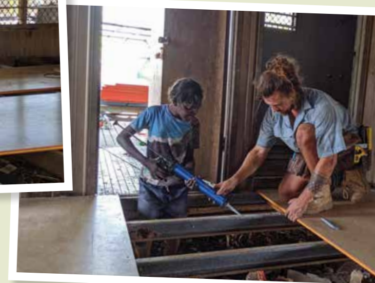
Mahalia helping to glue down the new floor in the house with volunteers from the Fair Tradies.
